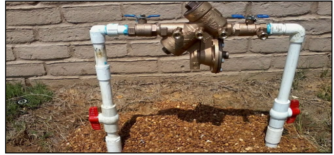
Example Installation of Irrigation Backflow Preventer
